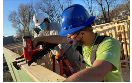
Trained staff and crew leaders supervise home construction, with volunteers and future homeowners contributing most of the labor.
