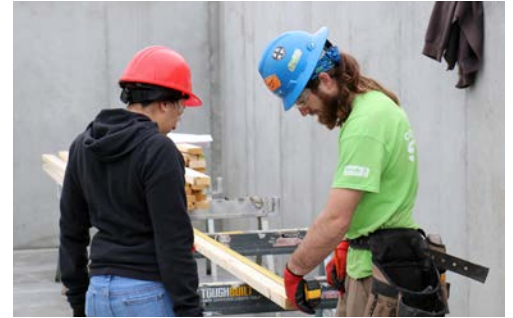
Trained staff and crew leaders supervise home construction, with volunteers and future homeowners contributing most of the labor.
